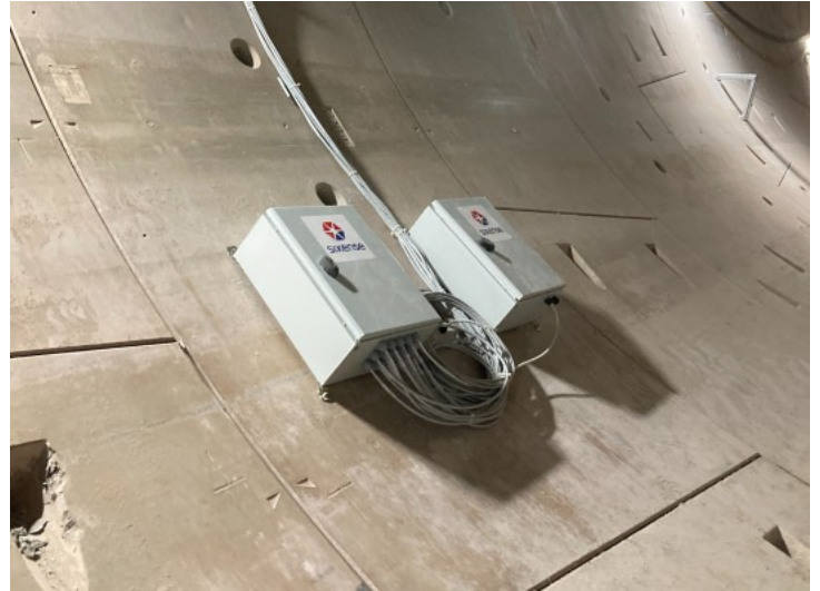
Tunnel Datalogging Enclosures
