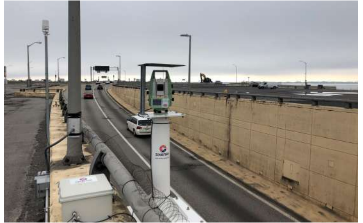
Cyclops - AMTS installed on site
